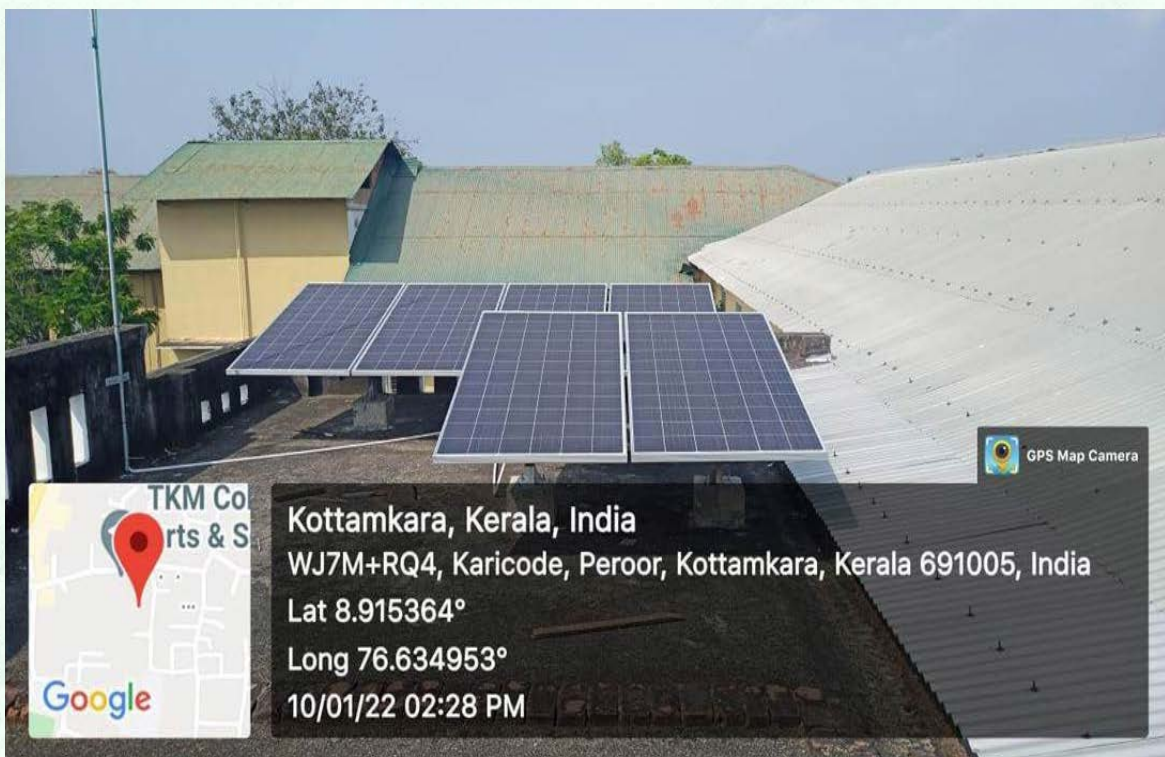
Solar panel systems
