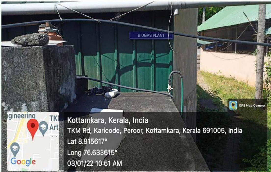
Biogas plants have been installed in the campus to convert the food waste generated into Biogas
