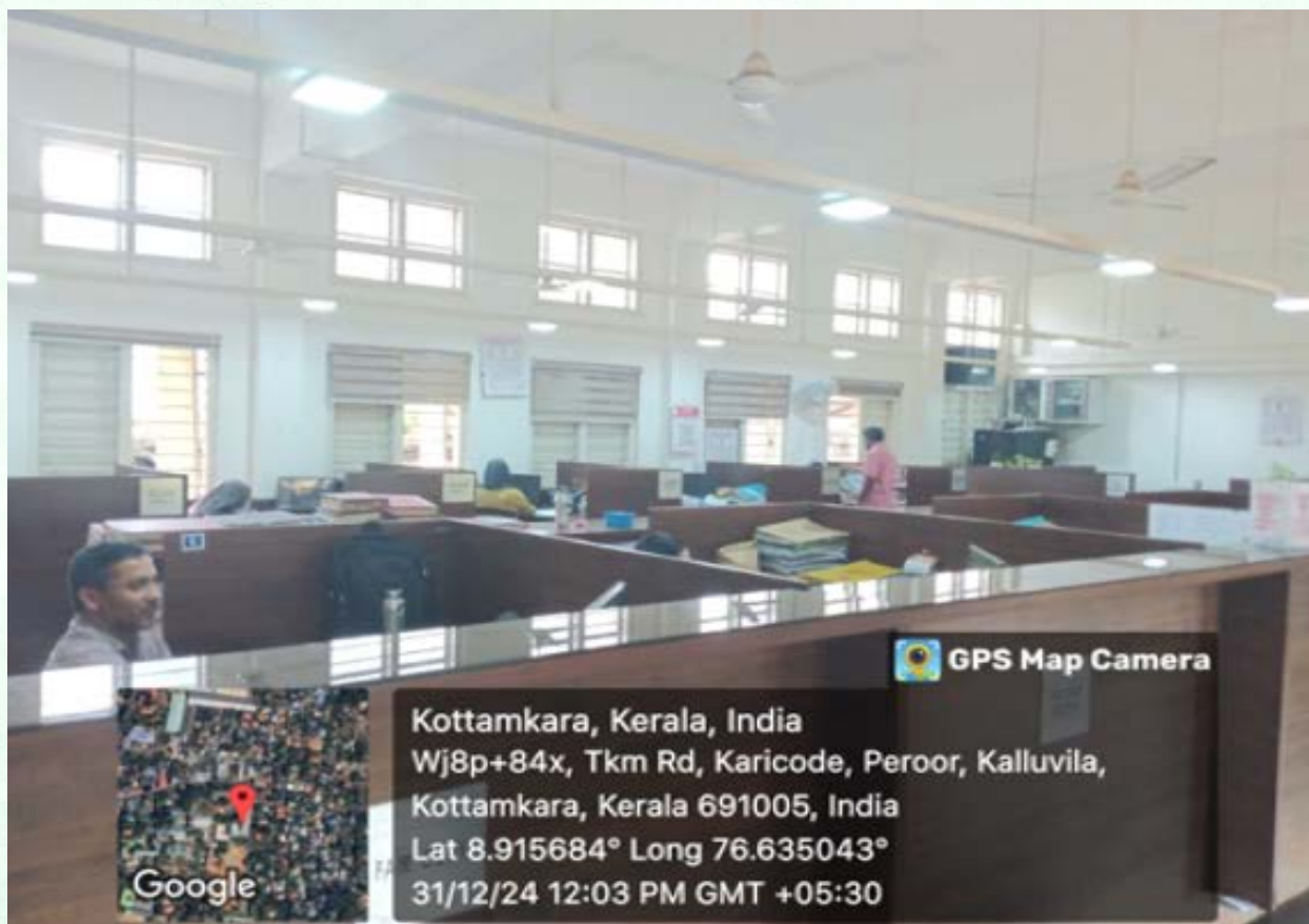
LED bulbs and LED tube lights are in the campus office
