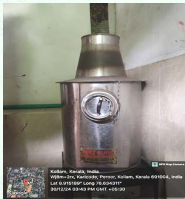
College has installed incineration unit in the campus for hygiene and proper sanitation
